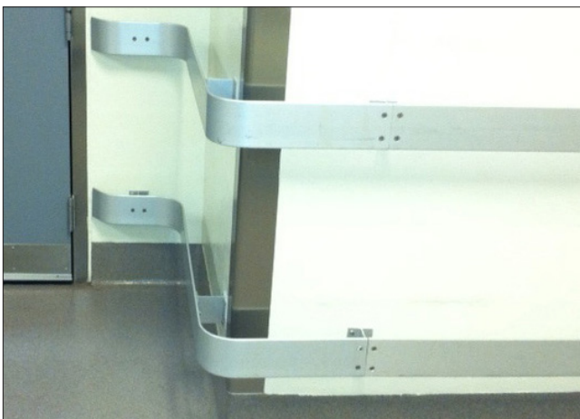
Figure 4.3.3.5 ARF Wall Protection
